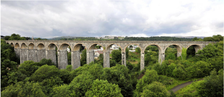
Viaduct at Cefn Coed-y-cymmer. It was built in 1866 to carry the Brecon and Merthyr Railway across the River Taff. (Courtesy: Ray Jones via geographic.org.uk)
